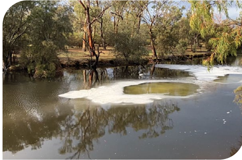
Image above: Artificial oxygenation of the Swan River at the Caversham oxygenation plant
